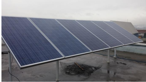
Figure 1. The installed PV system
